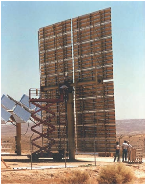
Figure 2.4 ATS fourth-generation prototype (148 m 2 ) from the USDOE large-area heliostat development program (1985–1986) (SANDIA).
