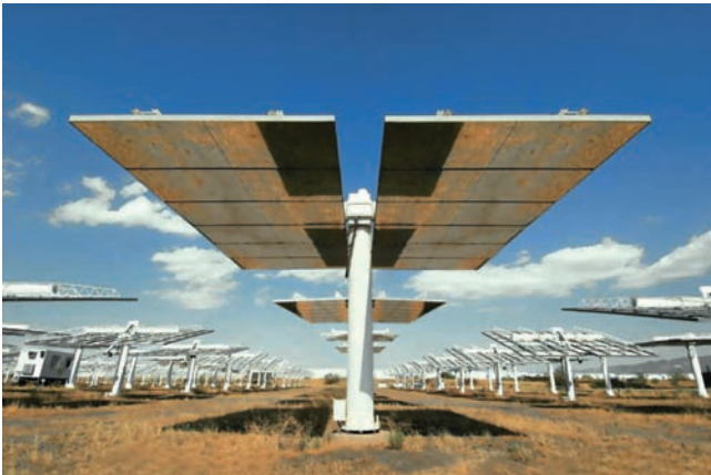
Figure 2.8 The heliostat field in front of the CESA 1 Tower (Almeria, Spain) (Photo DLR).
