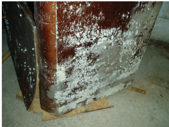
Figure 1.2 White mold on damp furniture wood in the basement, after rainwater penetration.
